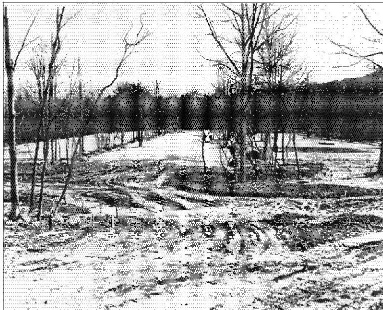
Figure 71: Catoctin RDA, Manor House Day Area, parking area under construction, ca. 1938. Source: Matthias C. Huppach Collection, Catoctin Mountain Park files.
