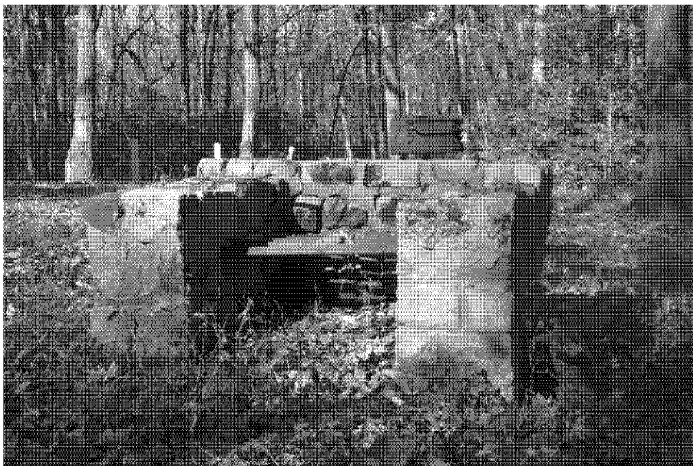
Figure 91: Functioning fireplace, Ridge Picnic Area, Fort Dupont Park, 2004.
