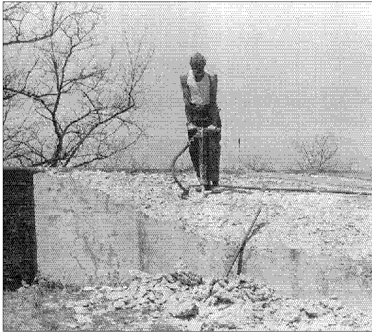
Figure 61: Camp NP-4-MD Enrollee Demolishing Concrete Wall at Fort Washington, c. 1941. Source: RG 79-CCC, Still Picture Branch, NARA.
